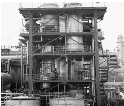
Installation de transformation de chaleur de 5MW – X. Ma, J. Chen, S. Li, Q. Sha, A. Liang, W. Li, Application of absorption heat transformer to recover waste heat from synthetic rubber plant
